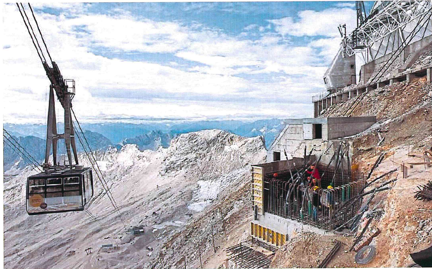
An existing cable car for skiers passes the construction site for a pylon for the new cableway.
