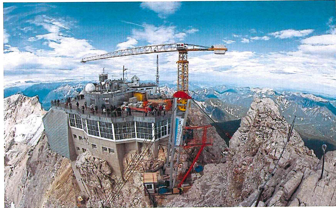
The existing restaurant and viewing platform, left, atop the Zugspitze. At centre is a crane and an especially constructed cargo cableway to haul building materials to the top of the 2,962m mountain in the Alps.
